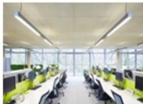
LED Lighting/ Daylighting/ Motion Sensors
